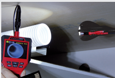
Ventilation inspection and servicing
